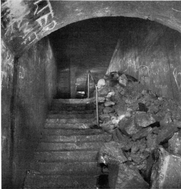
Cannon Road car park entrance. This is one of the few remaining access points into the tunnel network. There is a securely locked manhole cover at the top of the ladder on the left.
